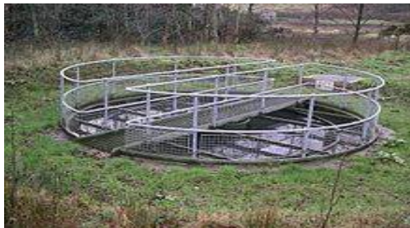
Figure: 3 Secondary clarifier at a rural treatment plant.
