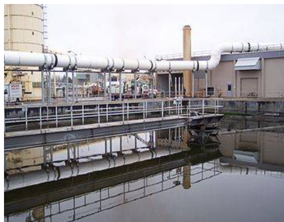
Figure: 2 Primary treatment tanks
